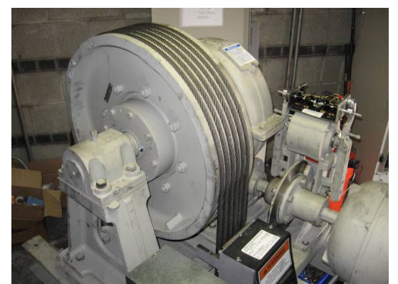
New jail elevator geared machine that raises the elevator car.
