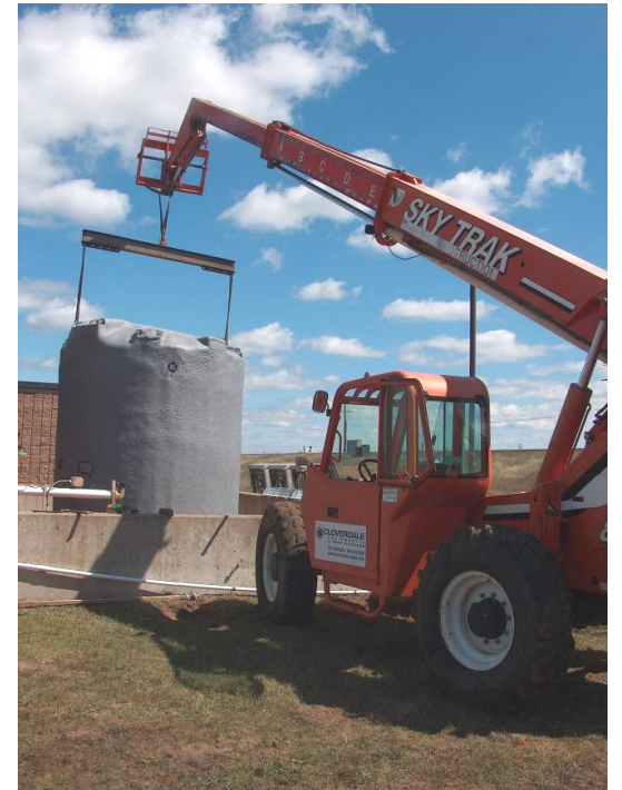
New ferric chloride storage tank being installed for the RI System at Wastewater
