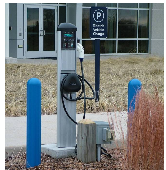
Electric vehicle charging station
