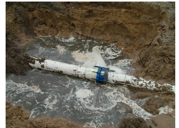
Irrigation pipe failure in Field 51 at Wastewater
