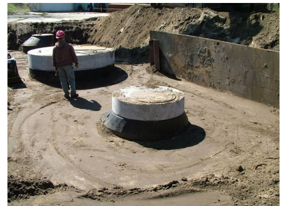
City of Muskegon wastewater meter installation
