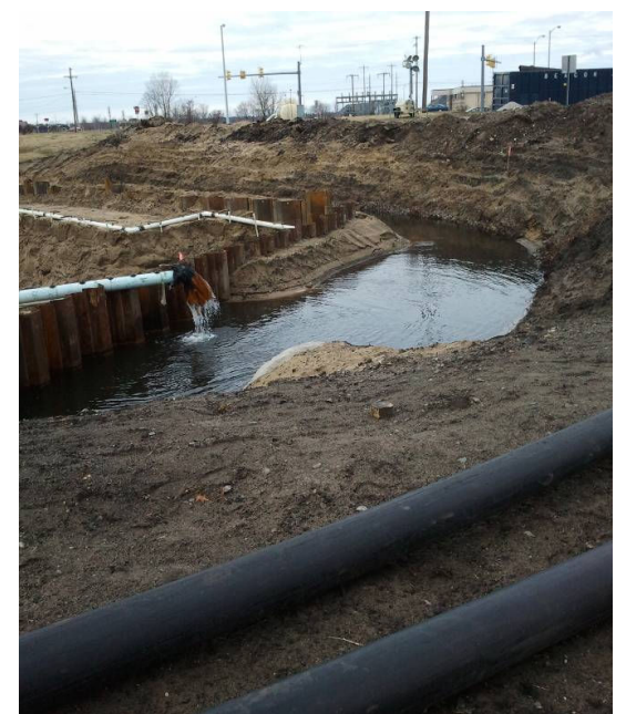
Replacement of a 72" culvert on Yuba Street that runs under one of our Wastewater lines
