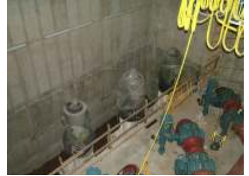
New C Station pumps and piping
