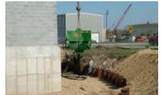
New C Station block wall done, backfill progress, and pulling the sheet piling
