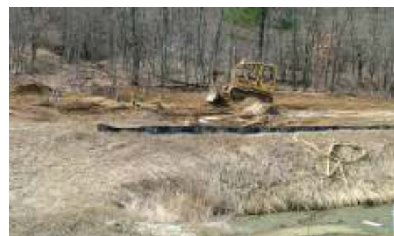
Grade work where the new Sullivan Pump Station will be installed across the ditch from the existing station
