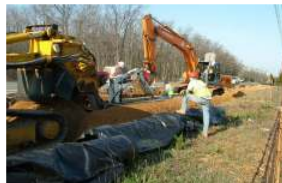
20-inch ductile iron force main being installed along Apple Avenue between Laketon and Sullivan Pump Stations
