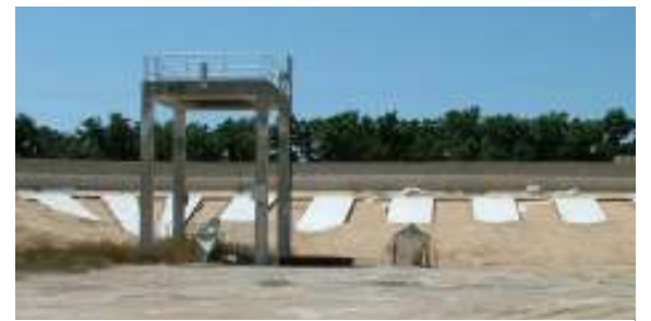
The new inlets to Cell #1, the new cell outside wall, and side slope concrete have been completed
