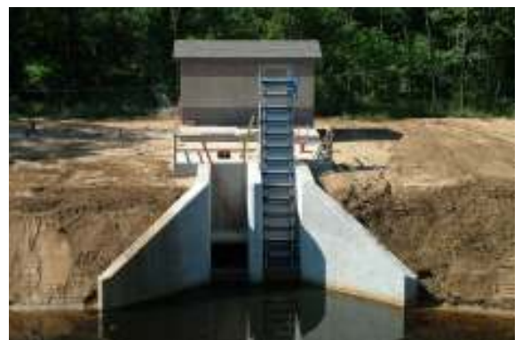
Trash rake at new Sullivan Drainage Station
