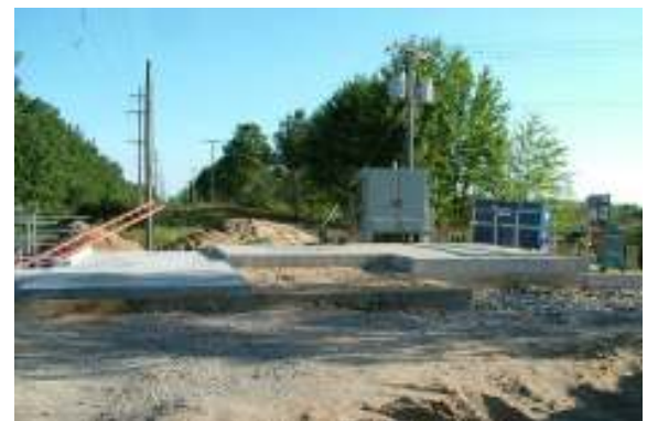
The rebuilt Laketon Station site changed with the addition of submersible pumps
