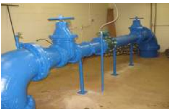
New main meter at Ottawa Street Metering Station
