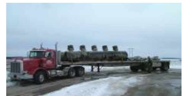
Old pipe header removed from Pump Station #3 in preparation for strainer installation next spring
