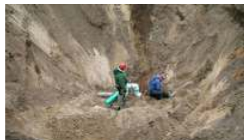
Contractor installing PVC tubing in RI drain tubing to permit direct sampling
