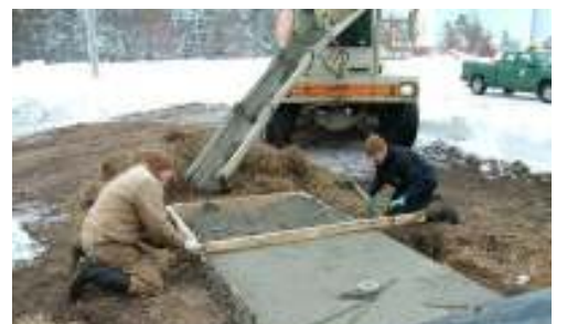
Our Parks crew pouring a pad for a generator at Fleet Maintenance
