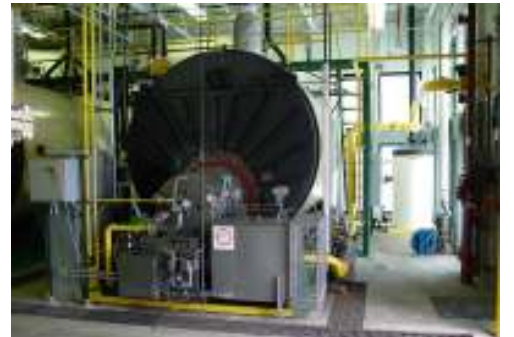
Boiler at Sun Chemical where our landfill gas is used
