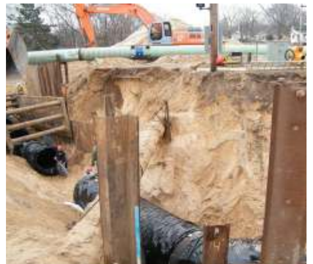
Installing the last few Wastewater System 60-inch restrained joint pipes with the bypass line in the background
