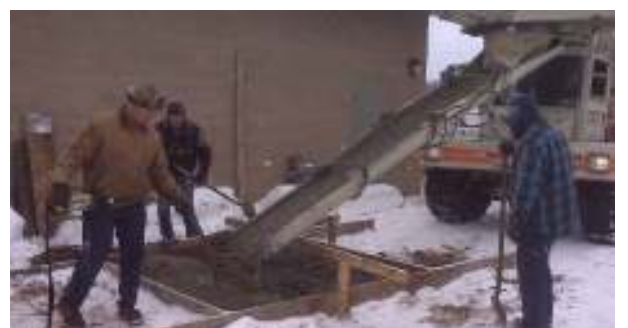
Pouring the concrete base for the new 80-foot antenna at the Quarterline Road Pump Station
