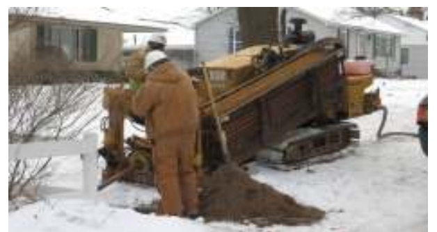
Directional boring an 8-inch water main under Center Street and over the Holland Drain culvert
