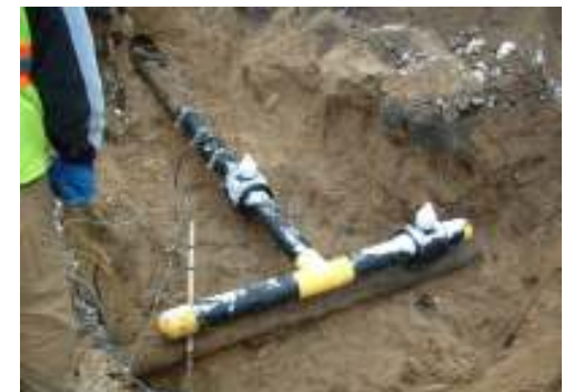
Landfill gas lead into Sun Chemical
