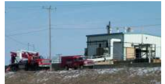
Electrical contractor removing primary power from the Pre-Aeration Building prior to its demolition
