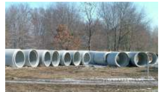
Concrete pipe stored on the Wastewater Plant site for crossing the interception ditch with the 60-inch force main
