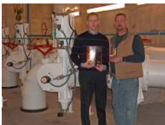
Mark Eisenbarth, County Project Manager, poses with Northwest Kent Supervisor Mark Decat in front of some of the award-winning process piping at Lift Station C
