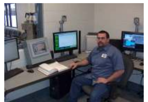
Collection System Operator Rodney Holland in new C Station control room
