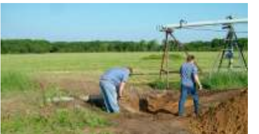
Patrick Pastor and Shane Sietsema with the old pivot pad of Rig #9 removed
