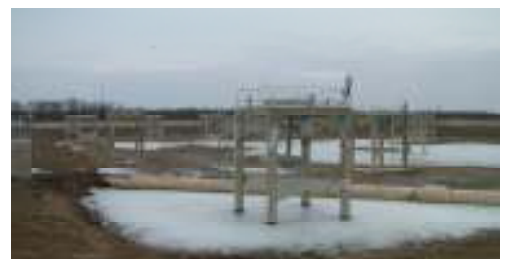
Cell #1 ready for platform work prior to installation of rebuilt mixing equipment
