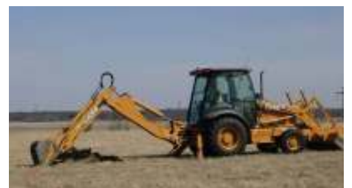
Grizz digging the cover off the cap liner so that soil borings can be taken on the fly ash hill for the wind turbine project
