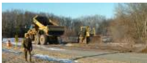
40-yard off-road truck unloads sand to help staff repair erosion on the Wastewater site
