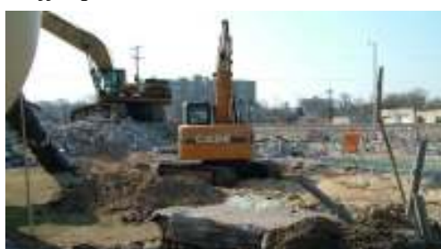
It's gone! The above-grade demolition of our old Lift Station C is nearly done
