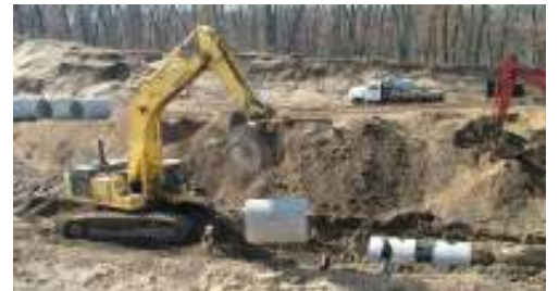
K&R laying 60-inch concrete culvert in the interception ditch where the 60-inch force main will cross it
