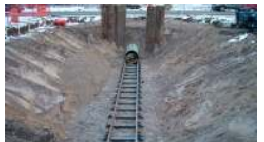
Set up for boring under Apple Avenue for Laketon Station to Sullivan Station pipeline
