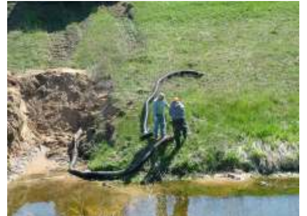
Antione and Ron repair a washout in one of the RI System ditches
