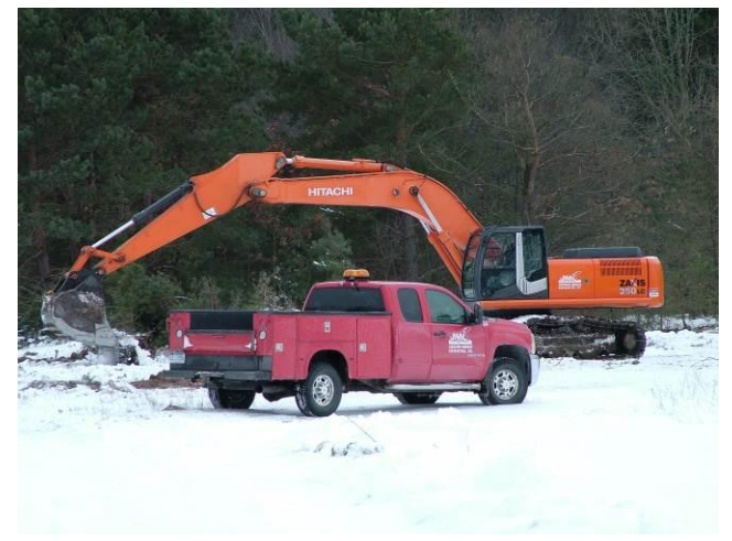
Prep work is underway on the flow-through marsh project on the Wastewater site
