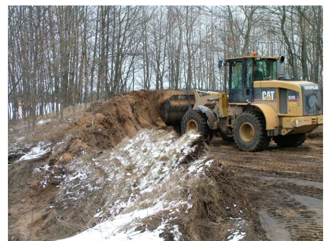
Ron Glover works on moving dirt and clearing trees as part of the marsh project
