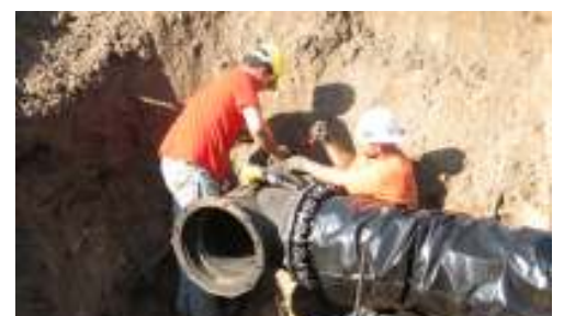
Laketon Township Contract #2 water main installation at Pennsylvania Avenue and Memorial Drive
