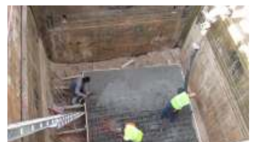
Construction crew pouring the base to Laketon Township's Green Creek sewage pump station
