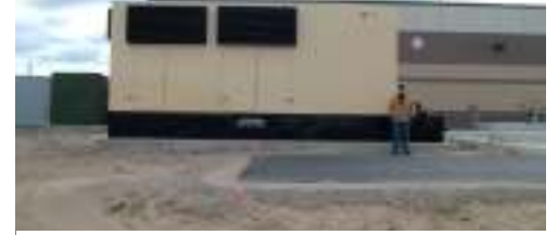
Supervisor Mike Barry standing by the 1,500 KW generator in back of our new C Station – it will run two of the 600-HP motors simultaneously
