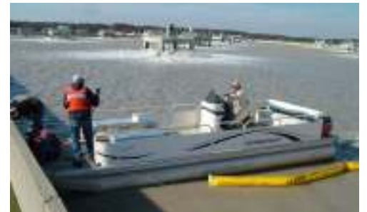
Installing a floating boom in Cell #2 to keep trash from overflowing the lagoon
