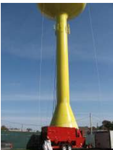
Humidity control was maintained on the inside of the Fruitport Water Tank while the contractor was doing sand blasting
