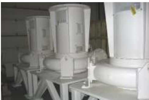
New Lift Station C pumps
