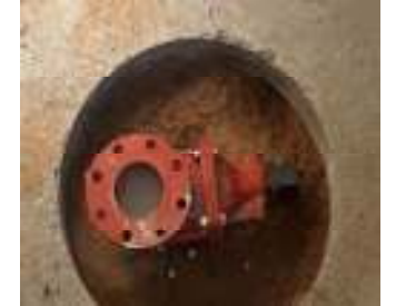
A 4-inch hot tap on our 66-inch force main for fiber optic monitoring
