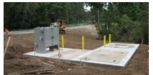
Sewage lift station near Horton and Glenwood in Laketon Township
