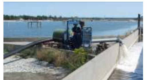
Millions of gallons per day being pumped from Cell #2
